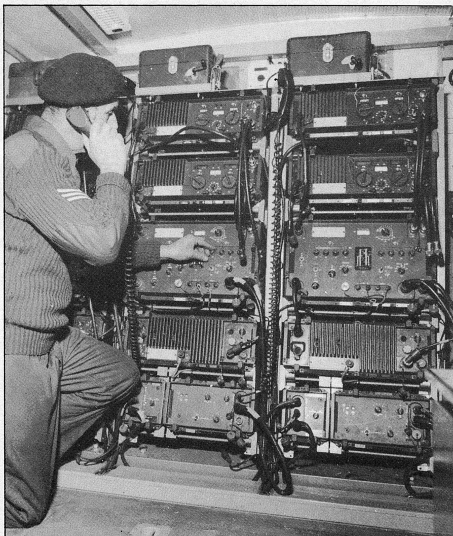
5 A typical Triffid installation: three stacks of equipment providing relay operation plus standby
