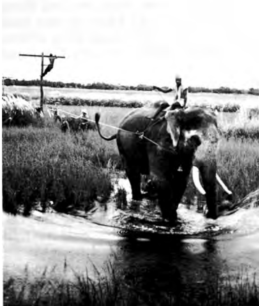
ELEPHANT DRAWS WIRE TAUT during pole line construction near Shampur, India. 31st Signal Construction Battalion.
